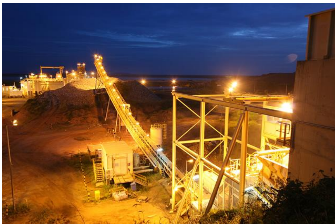
Stockpile feed conveyor CV-0. Typical installation of out feed ore handling from a ROM cone crusher.
