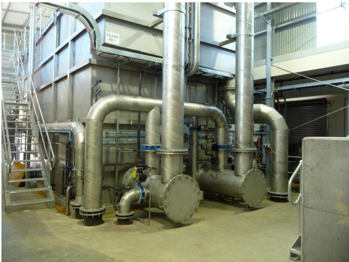
Raw water treatment plant DAF filter constructed from high grade stainless steel.
