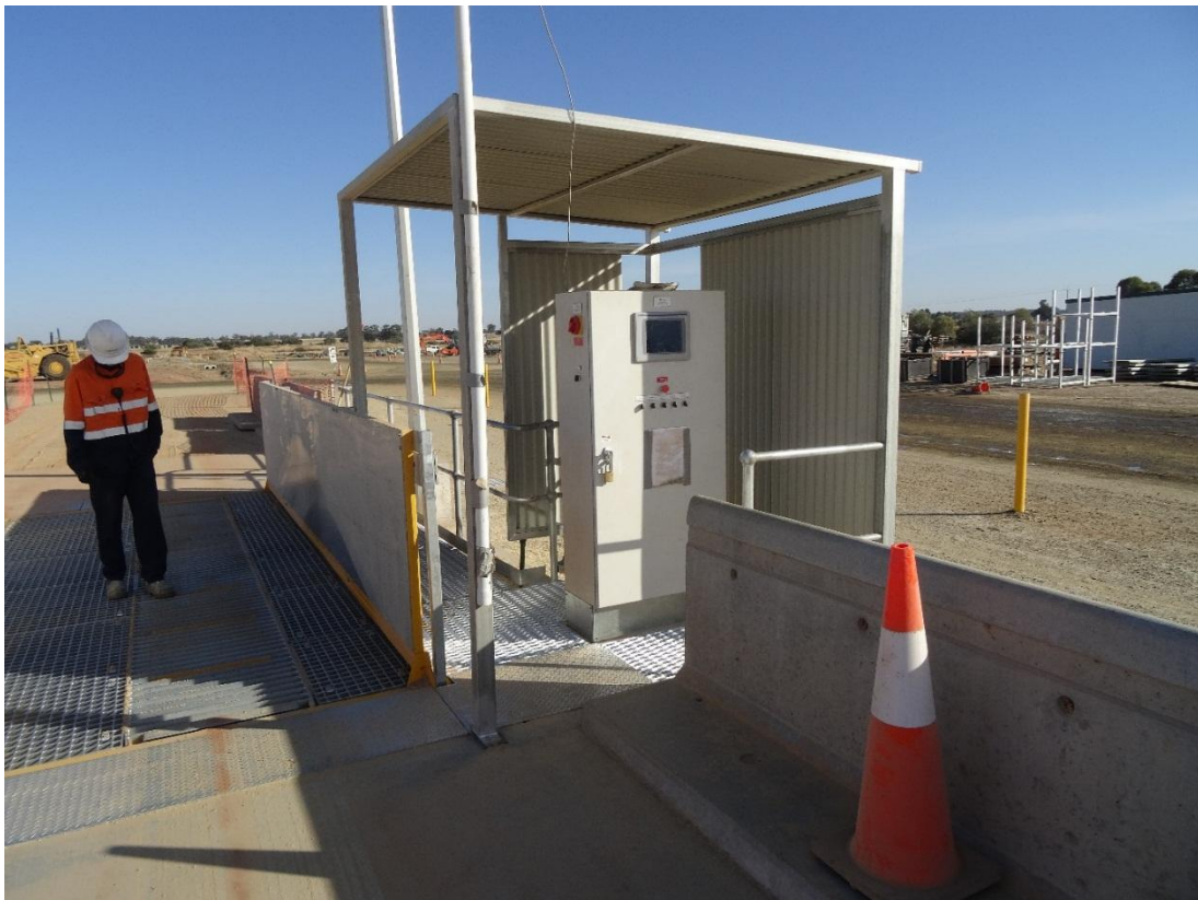
600 TPH DOH (drive over hopper) West Wyalong NSW
