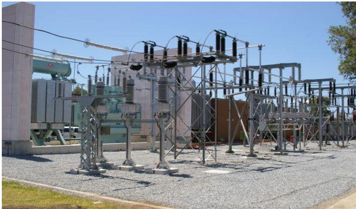
Burwood 132kV to 22kV zone substation showing VT's in the foreground followed by isolation switches and circuit breakers.
